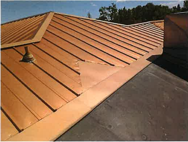
Aging pipe boot needs replaced. This is a likely leak location.
