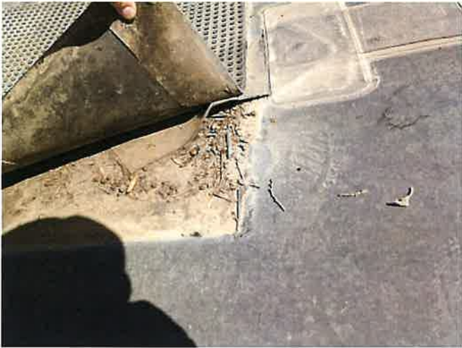
Walk pad peeling up flashing.
