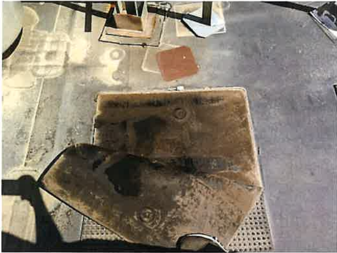
Additional walk pad needing reattached.
