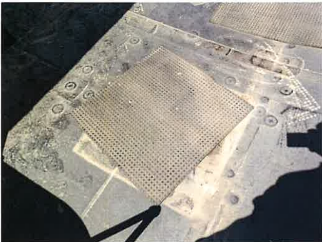
Detached walk pad. Needs reattached.
