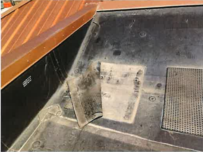
Detached walk pad. Needs reattached.
